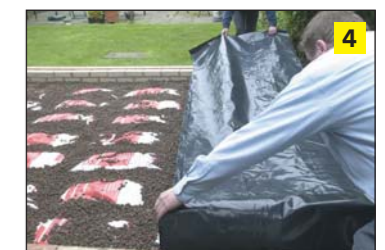
Step 4 Lay a 1200 gauge damp proof membrane over the insulation fill. The insulated floor is ready to receive the concrete slab.
