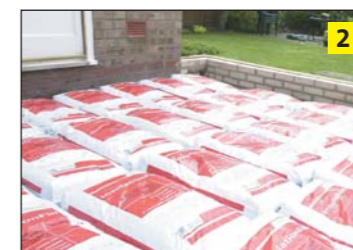
Step 2 Continue to lay bags side by side to cover the floor area. If a second layer is needed, lay in a brick bond pattern.
