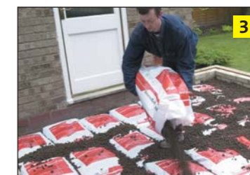
Step 3 Once at the required depth, use loose material to fill the holes between bags and level off.
